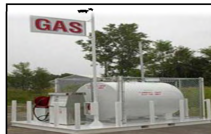
Full Code Fueling System
