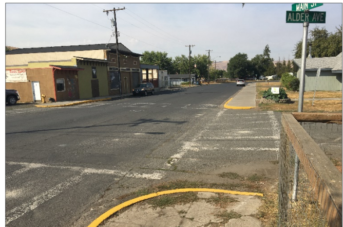
Figure 5 – Intersection of Main Street and Alder Ave showing signs of deferred maintenance. Image Credit: Jason Espie
